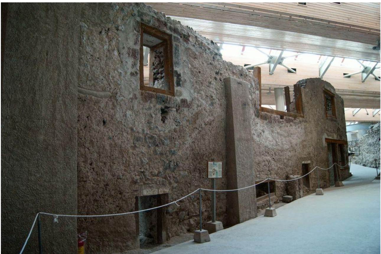
Figure 2: Different forms of window in southwest face of West House in Akrotiri (Image Copyright: Rianca Vogels)
